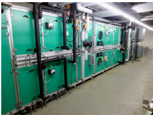
A specialised air ventilation system enables the circulation of external air into the interior of the building whilst ensuring a pressure gradient between the different rooms.
